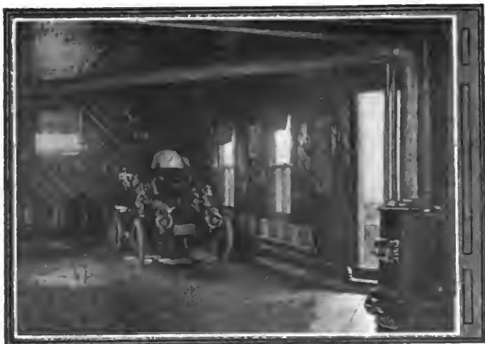
Elaborate and Efficient Heating Plant in Paterson Garage
